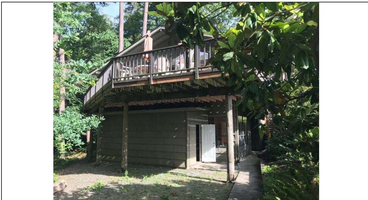
Plate 2. Proposed new bay on north side of basement level planned within footprint of existing storage room below deck, facing south.
